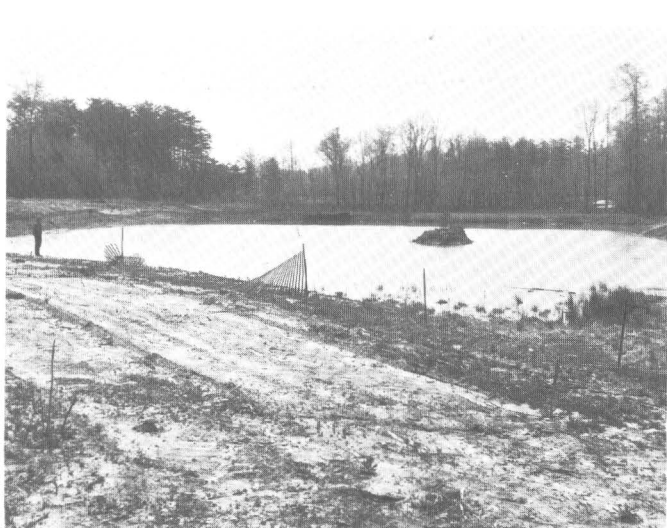
FIGURE 19.—Large sediment-stormwater management basin used to trap sediment before it can leave construction sites, Bel Pre Creek basin, 1974.
