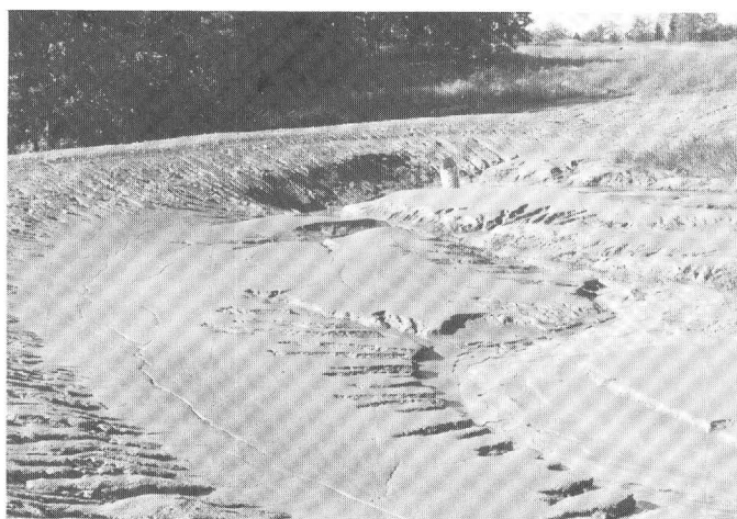
FIGURE 27.—Small sediment basin requiring maintenance.
