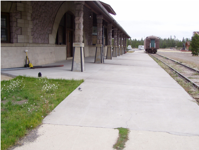
Looking east along the south side of the building at bench mark (near yellow GPS unit).
