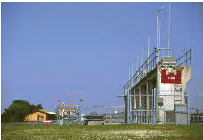
Figure 3. Flow regulator in Southern Florida Coastal Plain Ecoregion, part of water-control and -allocation infrastructure of Central and Southern Florida Flood Control Project, which was authorized by Congress in 1948 and constructed by U.S. Army Corps of Engineers, thereby ensuring continuation of urban and agricultural growth after World War II.
