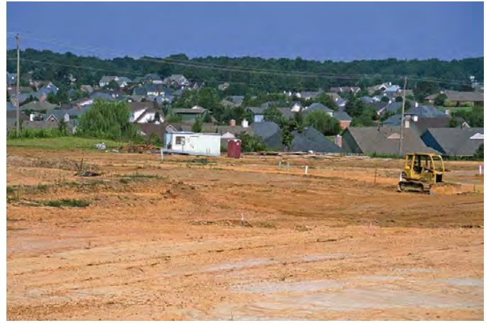
Figure 8. Recently cleared site for new subdivision northeast of Memphis, Tennessee. Existing subdivision is in background.
