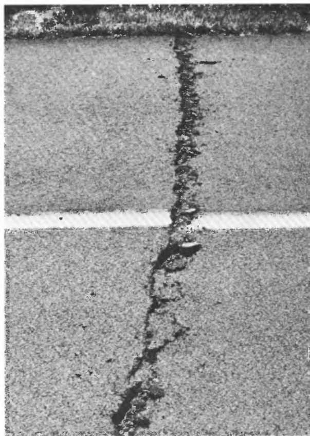
FIGURE 44.25.—Earthquake-produced crack across road at northwest entrance to Waldron Ledge Overlook. Chips of broken pavement indicate sides of crack were bashed together repeatedly. Photograph by J.B. Stokes.
