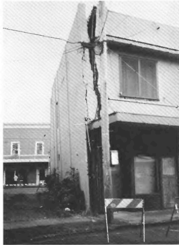
FIGURE 44.17.—Damaged commercial building in old part of Hilo. Side wall separated from main structure, leaving a gap at roof level of about 21 cm.
