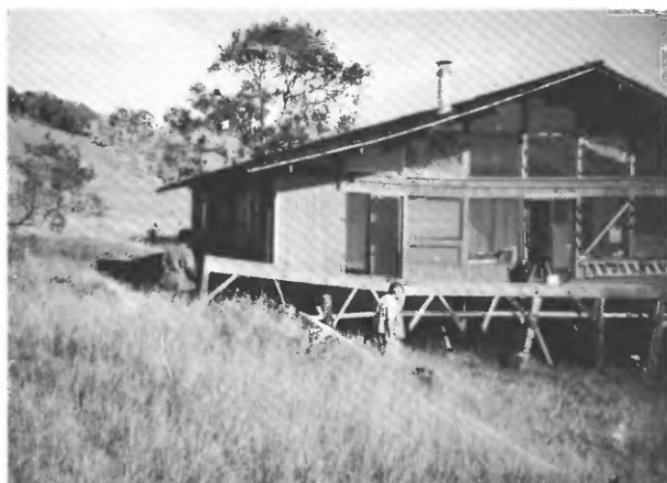
FIGURE 44.7.—House on Kapapala Ranch about 12 km east of epicenter was displaced 0.8 m northeastward during earthquake. Most supporting posts remained vertical, but those used to frame a basement room were tilted. Concrete foundation piers, partly obscured by grass, behind figure in dark jacket. Windows broken during earthquake are covered with plastic. Near clump of trees on hill behind house, small soil slips can be seen and broken branches strew the ground.
