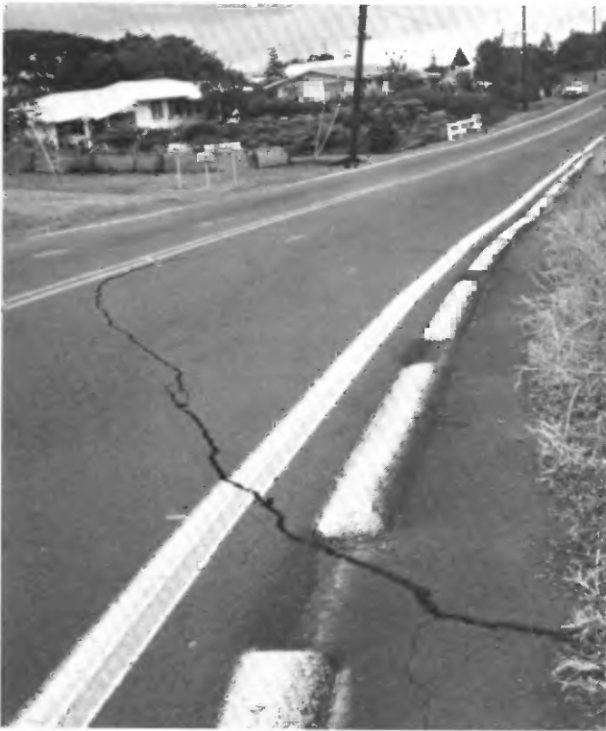
FIGURE 44.28.—Arcuate road crack along Kaumana Drive (fig. 44.15, area A) formed in November 1983 earthquake. Ground slopes downward to right. Houses were structurally damaged and water main was broken in area just out of photograph to left.
