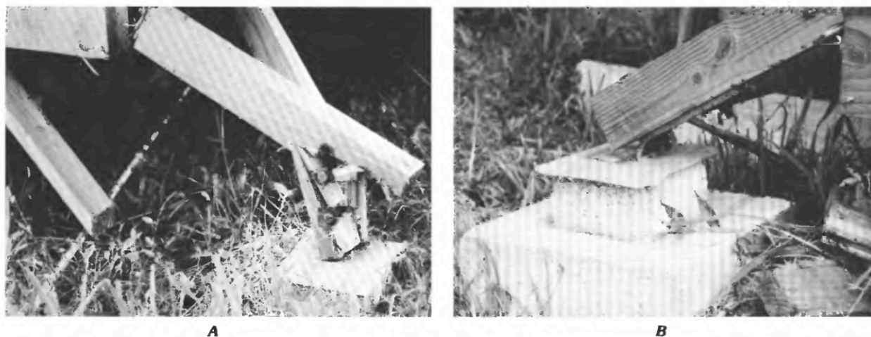
FIGURE 44.5.— Damage to a wood-frame house with post-and-pier construction in Wood Valley (fig. 44.4, locality b). A , Northeast corner post fractured where anchor bolts connected it to 0.5-cm-thick steel plate positioned on southwest side of post (away from the viewer). Concrete foundation block appears to have been poured as single unit around the steel plate. Post also was torn loose from house and from diagonal bracing when ground, pier, and post moved southeastward. B , Northwest corner post with steel plate on south side of post. The 0.5-cm-thick steel plate is bent at 45° angle. Photographs by E.T. Endo.
