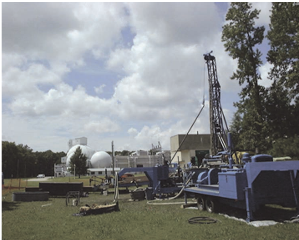
Equipment used to drill the USGS-NASA Langley corehole at the NASA Langley Research Center in Hampton, Va., in 2000. Photograph by E. Randolph McFarland, U.S. Geological Survey.
