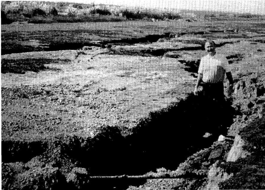
Figure 24.—Fissures, sand boils, and grabens associated with lateral spreading near northwest end of main runway at Oakland International Airport. Photograph courtesy of B.A. Vallerga.
