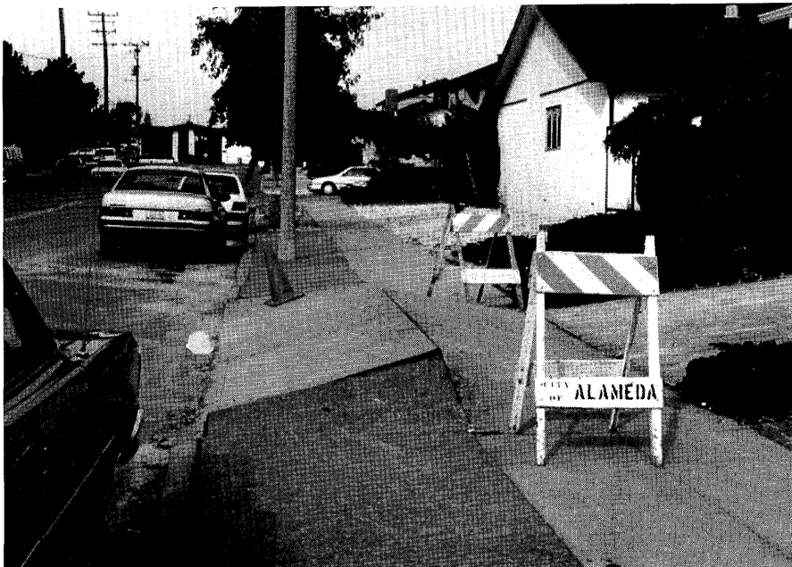
Figure 17.—Minor settlement and buckling of pavement at southwest edge of the Alameda (fig. 1).
