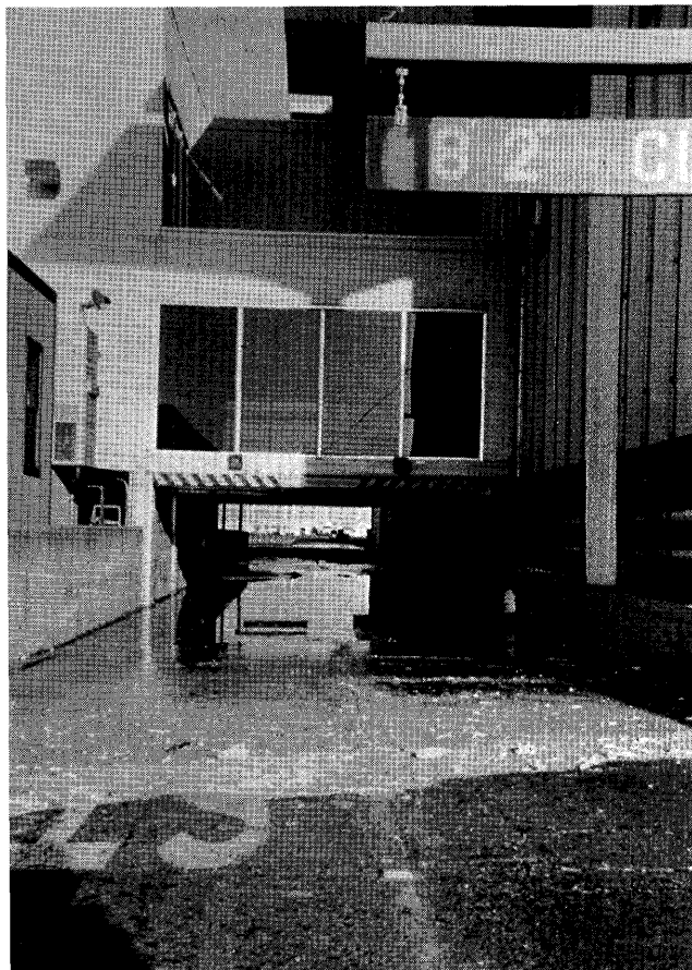
Figure 25.—Below-grade tramway, filled with as much as 1.8 m of extruded sand, at Oakland International Airport Terminal Building. Photograph courtesy of B.A. Vallerga.
