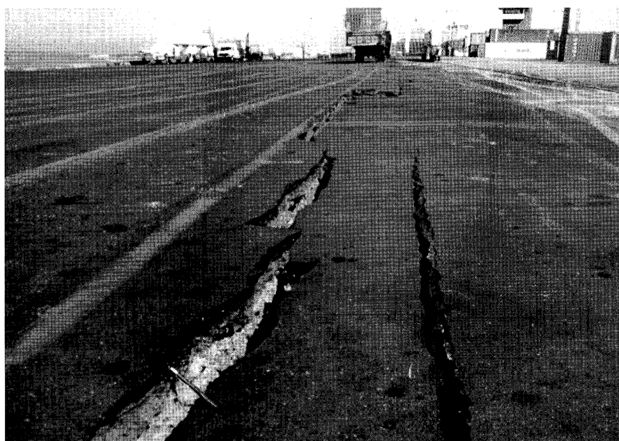
Figure 12.—Closeup of damaged pavement near boreholes POO7-5 and POO7-6 at Port of Oakland Berths 36 and 37 (see fig. 5 for locations), showing differential settlement, open fissures, and lateral spreading.
