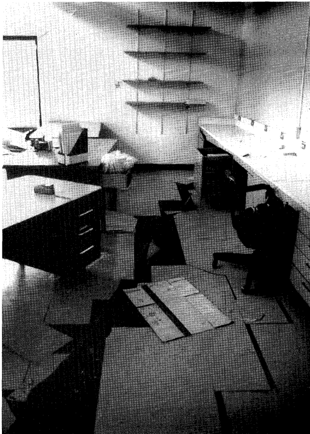
Figure 14.—Cracks in concrete floor in southern building of Moss Landing Marine Laboratory (fig. 11).
