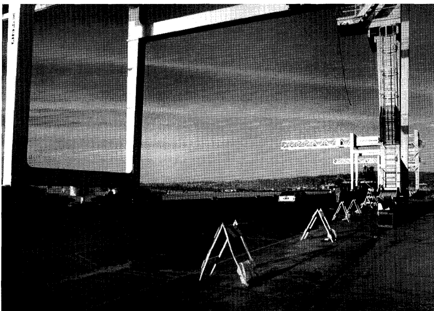
Figure 11.—Wharf of Port of Oakland's Marine Container Terminal at Seventh Street (viewed from Berth 37), showing shipping-container cranes, damaged pavement, and extruded sand.
