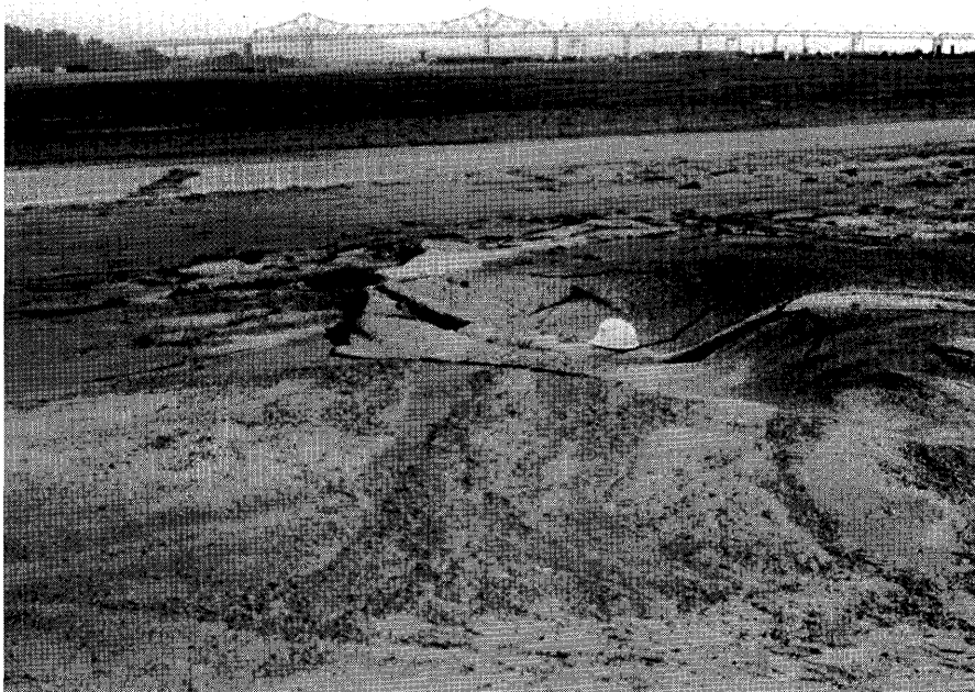
Figure 16.—Liquefaction-induced damage to taxiway pavement at Alameda Naval Air Station.
