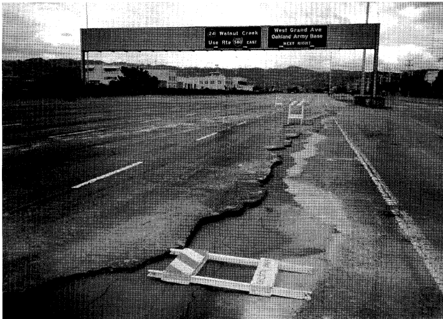
Figure 6.—Fissure in pavement caused by settlement in rightmost eastbound lane of Interstate Highway 80 west of San Francisco-Oakland Bay Bridge Toll Plaza administration building (visible in distance).
