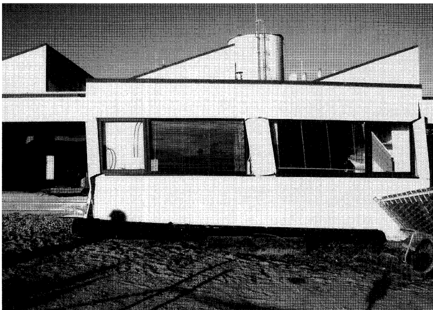
Figure 13.—Racking of southern building at southeast corner of Moss Landing Marine Laboratory (fig. 11).
