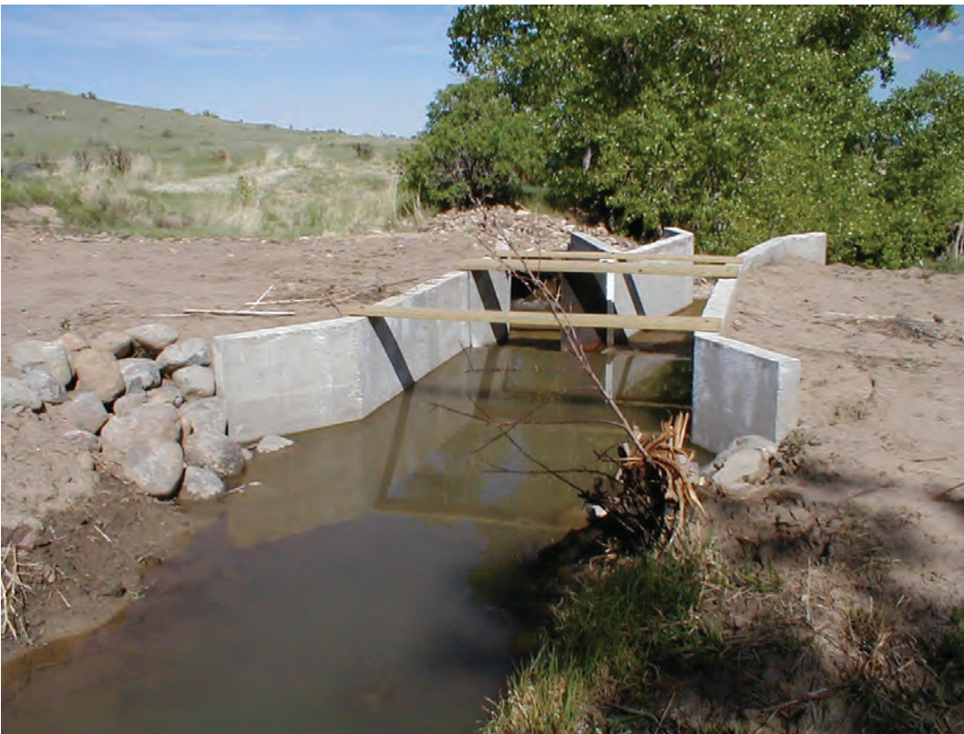
Figure 3. Splitter box located at measurement site SS07 on the Enlarged Southside Canal.
