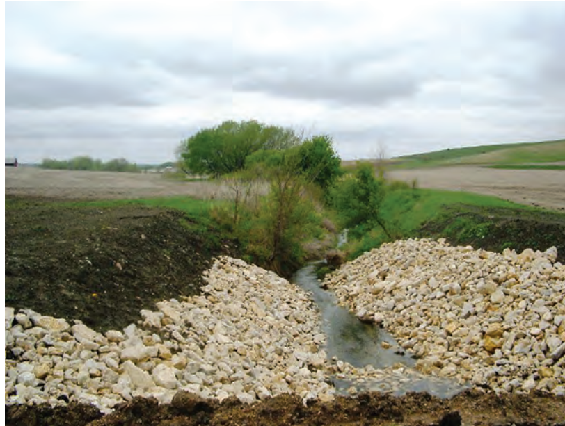
Figure A227. View looking downstream of culvert and road crossing, Stratton Creek near Washta, Iowa, May 5, 2003.
