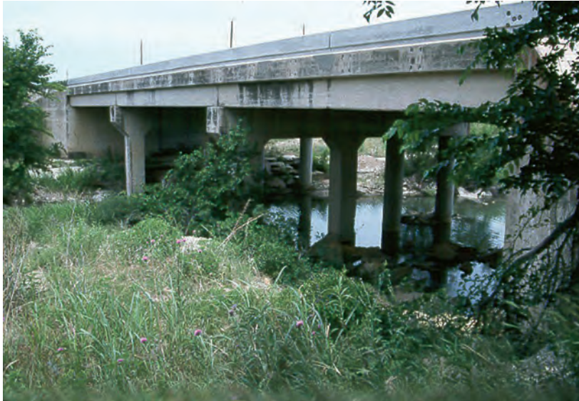
Figure A34. View from upstream side of State Highway 6 bridge, North Fork Hubbard Creek, near Albany, Texas, May 12, 2003.
