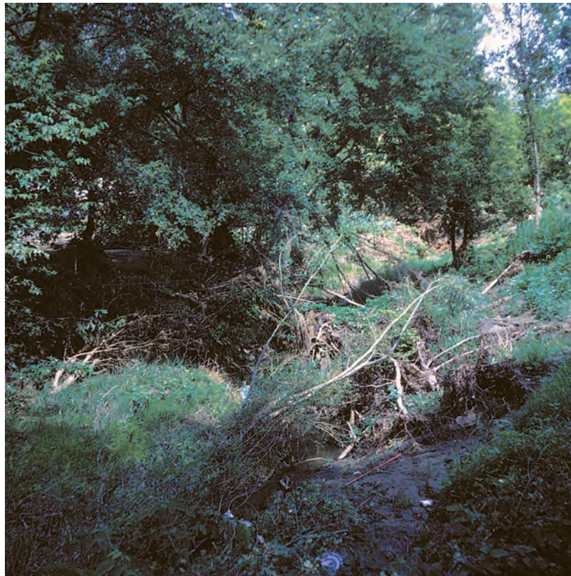
Figure A204. View looking downstream of cross section 2, Boney Branch at Rockport, Missouri, August 1965.
