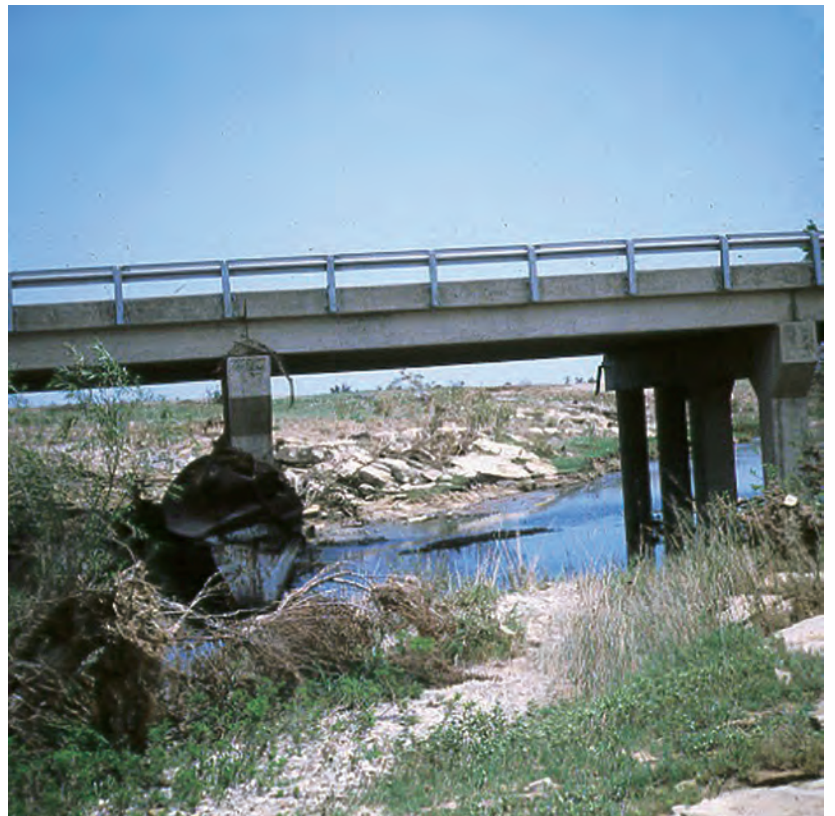
Figure A23. View at approach section to bridge at gaging station looking downstream at bridge and channel, North Fork Hubbard Creek near Albany, Texas, August 15, 1978.
