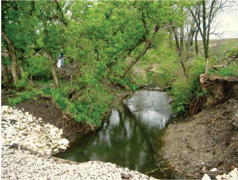
Figure A229. View looking upstream of culvert and road crossing, Stratton Creek near Washta, Iowa, May 5, 2003.
