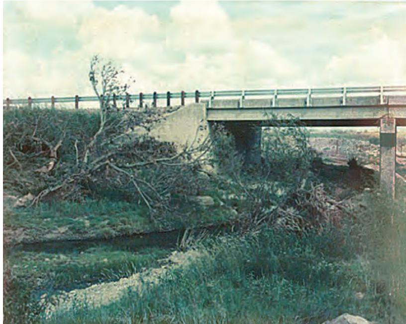
Figure A8 View of left abutment and upstream wingwall, North Fork Hubbard Creek near Albany, Texas, September 20, 1978.
