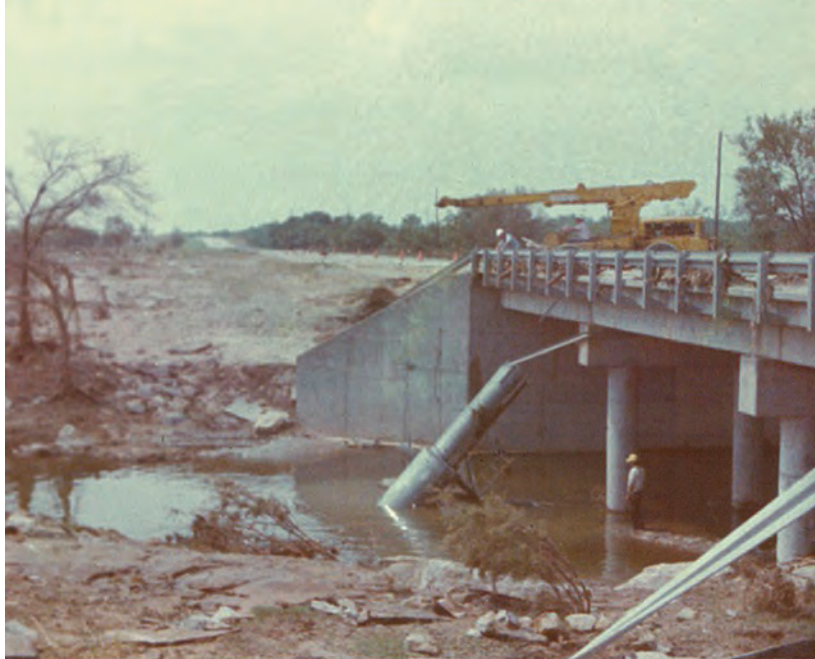
Figure A14. View of bridge and channel downstream from left bank, shelter and well being lifted out of stream, North Fork Hubbard Creek near Albany, Texas, August 10, 1978.
