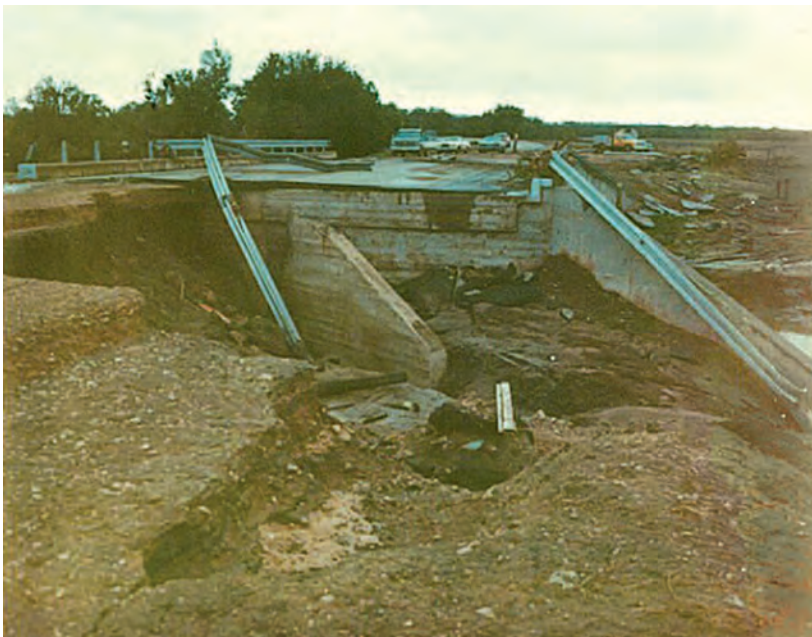
Figure A7. View from right end of bridge looking across bridge, North Fork Hubbard Creek near Albany, Texas, August 5, 1978. Flood of August 4, 1978, was about 2 feet over handrail.
