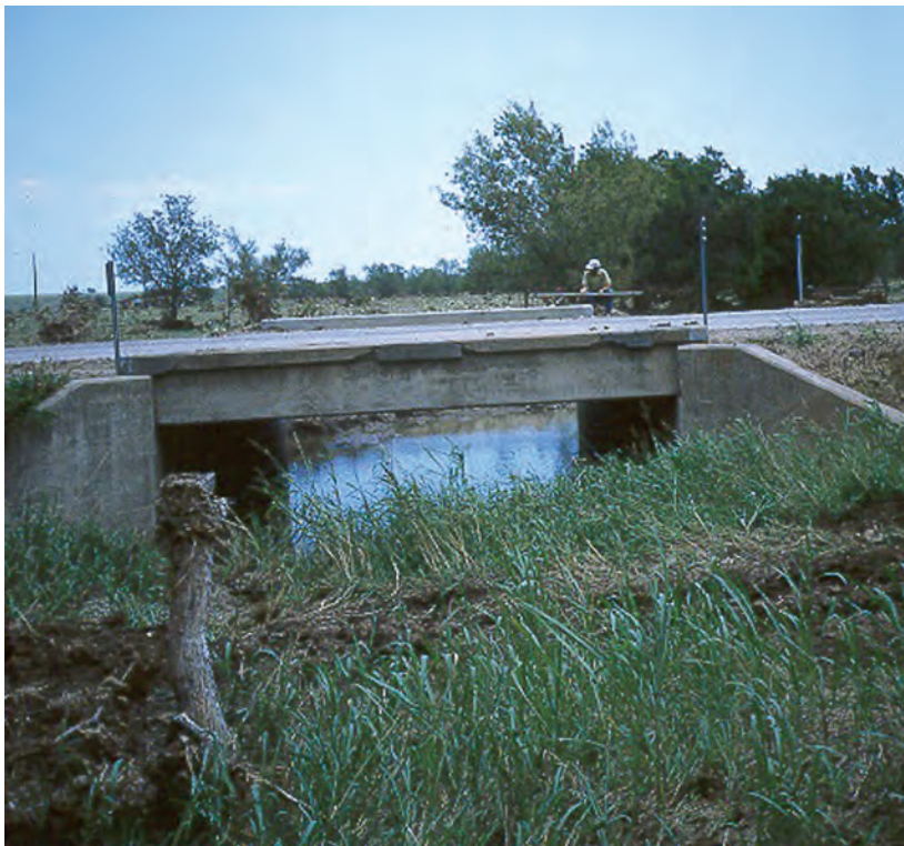
Figure A25. View at approach section of culvert looking downstream at culvert. Note flag in tree just above rod for elevation downstream of highway, North Fork Hubbard Creek near Albany, Texas, August 15, 1978.
