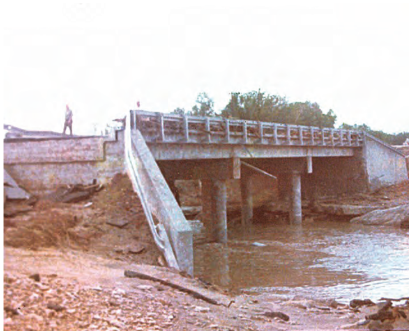
Figure A12. View of downstream side of bridge from right bank, gage shelter in center of stream, North Fork Hubbard Creek near Albany, Texas, August 4, 1978.
