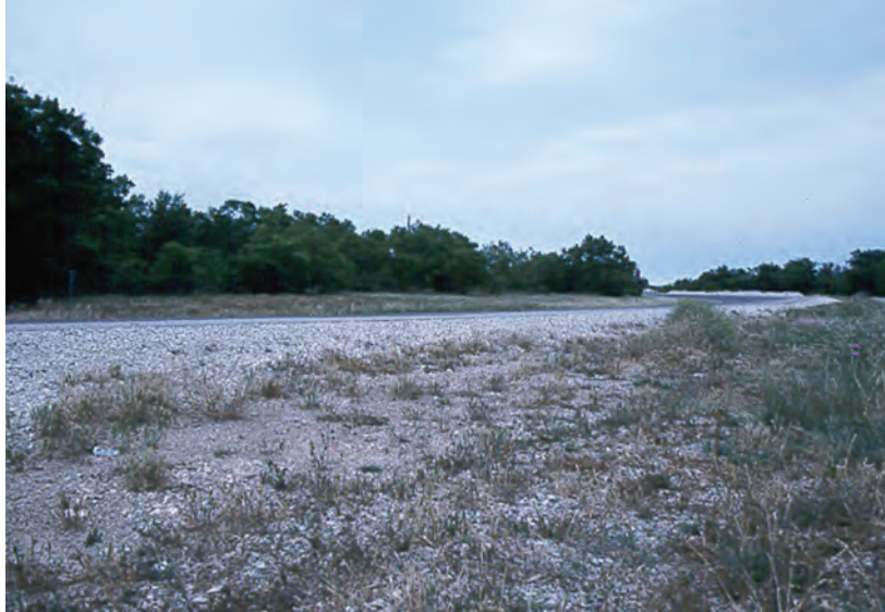
Figure A40. View looking upstream of downstream side of road near left end of bridge, North Fork Hubbard Creek near Albany, Texas, May 12, 2003.
