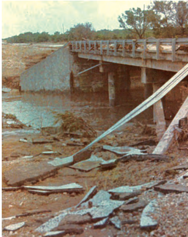
Figure A10. View looking downstream side of bridge from left bank, North Fork Hubbard Creek near Albany, Texas, August 4, 1978.
