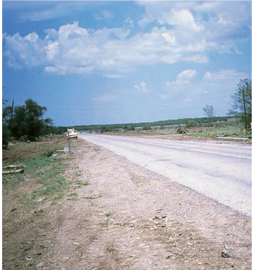
Figure A28. View about 100 feet to right of culvert on upstream shoulder looking slightly downstream and across to left bank. Rod held in approach section at high-water mark. The first string of trees is the main channel, North Fork Hubbard Creek near Albany, Texas, August 15, 1978.
