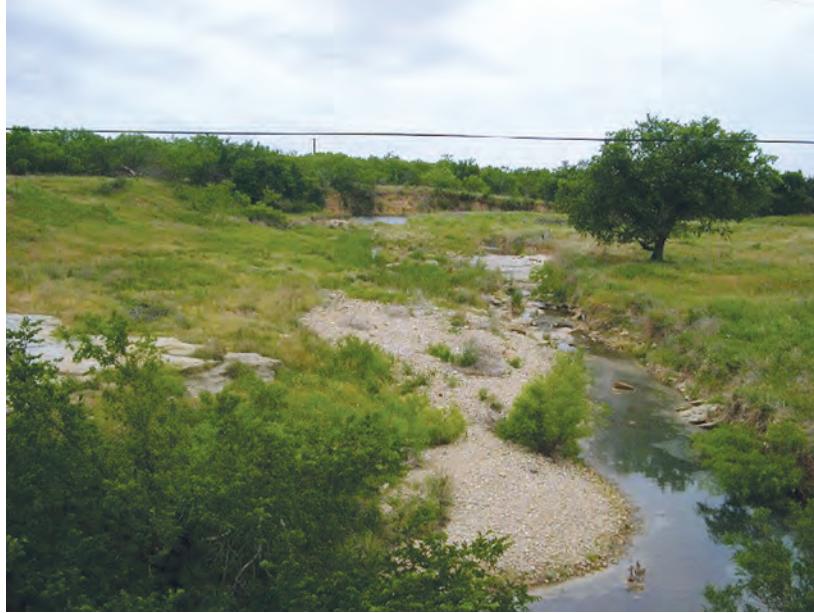
Figure A32. View looking upstream of bridge, North Fork Hubbard Creek near Albany, Texas, May 13, 2003.
