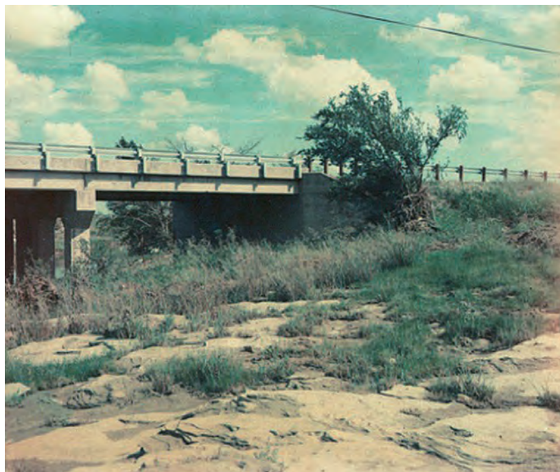
Figure A9. View of right abutment and upstream wingwall, North Fork Hubbard Creek near Albany, Texas, September 20, 1978.
