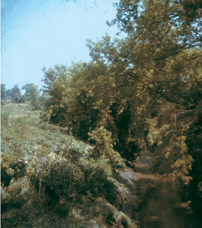
Figure A225. View looking upstream of culvert and road crossing, Stratton Creek near Washta, Iowa, August 1961.
