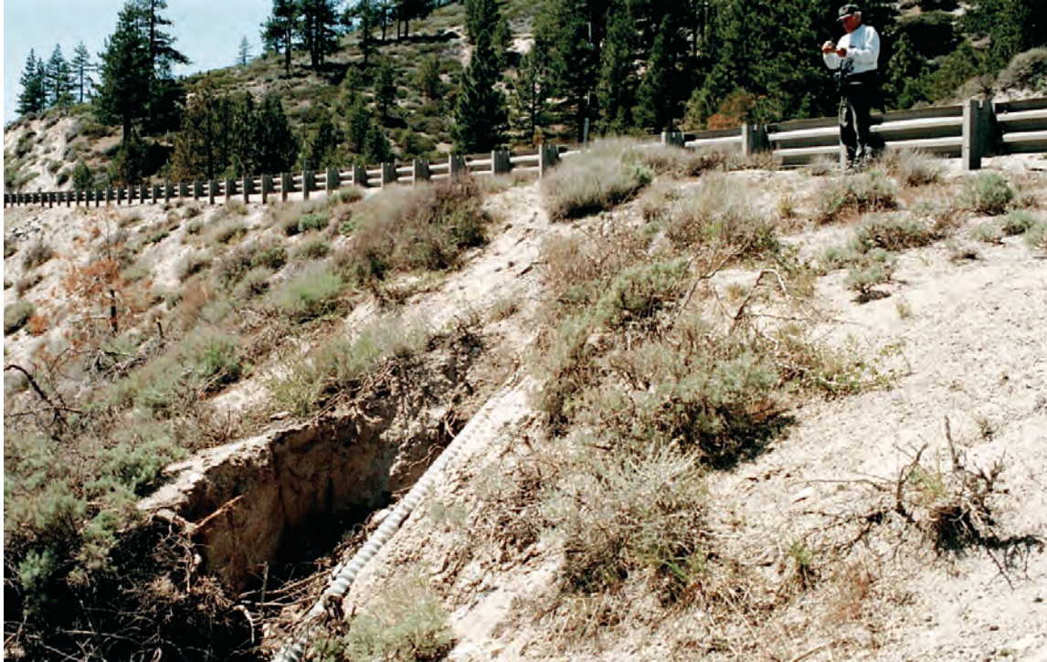
A. Gully headcut at drop culvert causing its collapse. Photograph taken by Jon Nowlin, May 2005.
