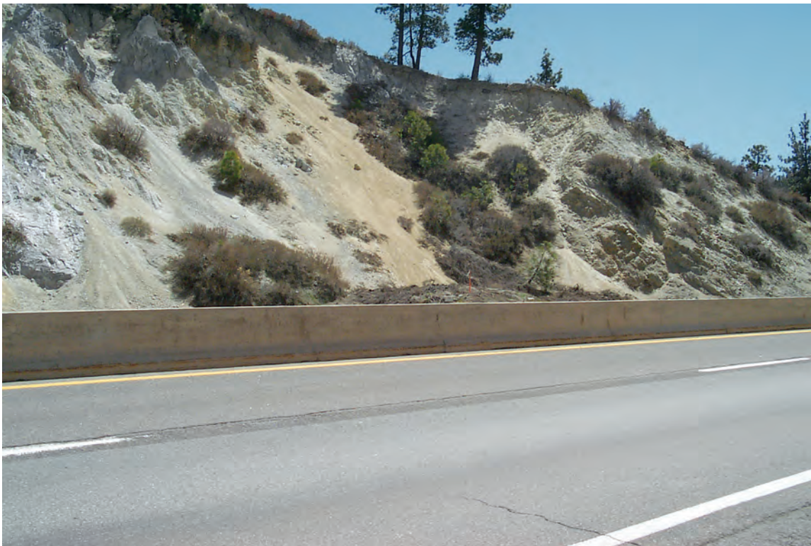
B. Land slumping along road cut. Photograph taken by Ralph Seiler, U.S. Geological Survey, April 18, 2008.
