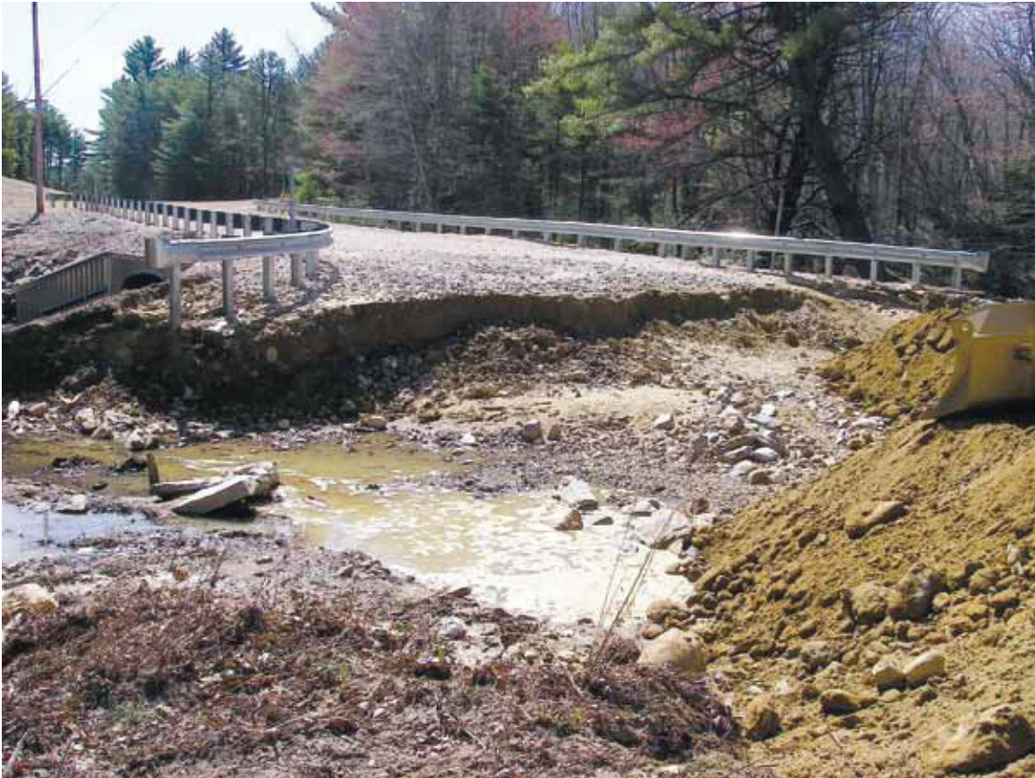
Figure 1. Keay Brook washout of Ridlon Road, April 2007, Berwick, Maine.
