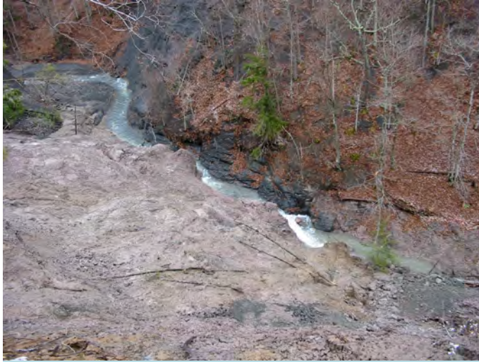
Slope failure which blocked Rattlesnake Gulf, late Winter, 2008, in the same area of the Spring 2006 slide pictured above.
