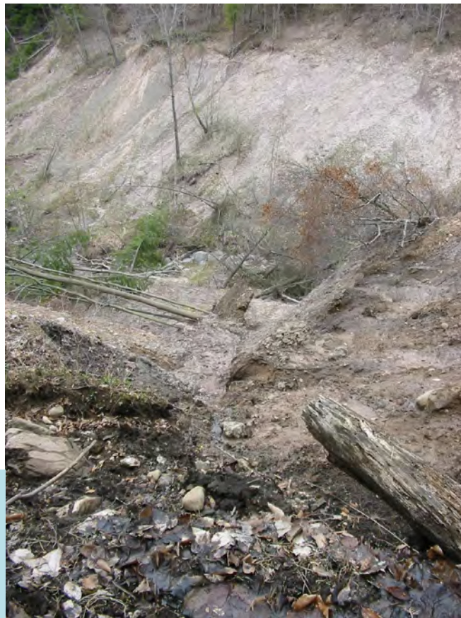
Toe of the slide area pictured above, showing debris flow and failure of opposite (north) slope of Rainbow Creek valley wall.
