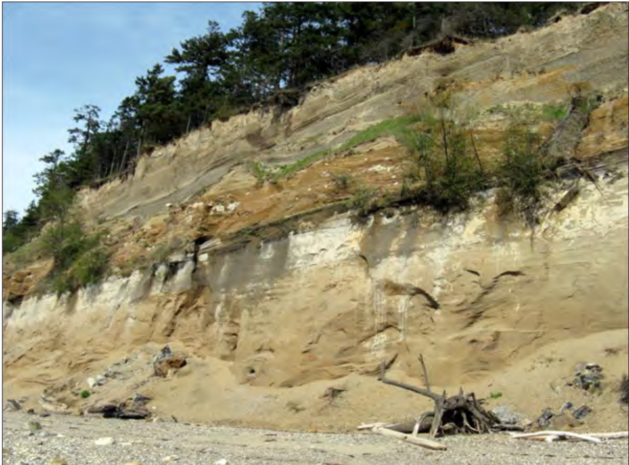
Figure 3. Eroding bluff on Guemes Island. 30-40-m high bluff consists of a diverse assemblage of Pleistocene glacial and glaciofluvial units and a wide range of sediment types, from silt to coarse gravel and boulders.
