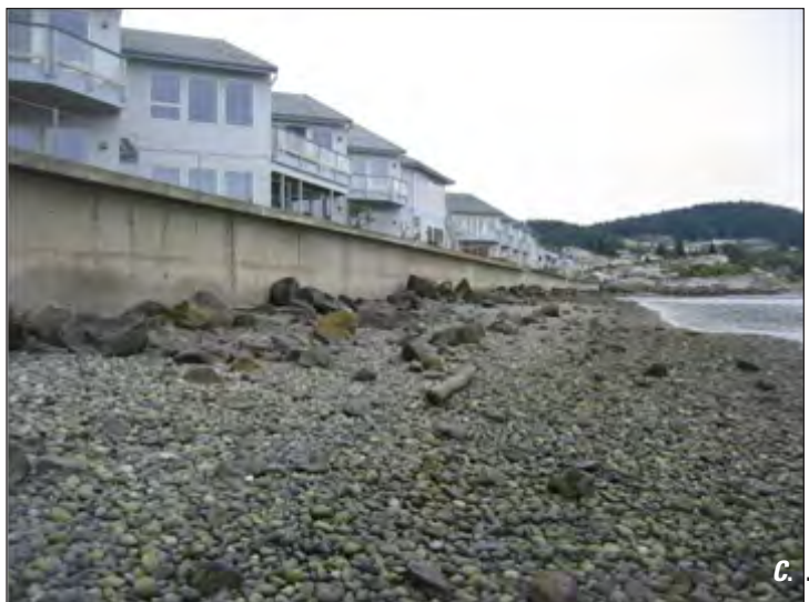
Figure 7. Typical examples of residential erosion control on Puget Sound. In each case, high tides would reach the seawall. (A) Rock seawall in Kitsap County. (B) Timber pile bulkhead on Camano Island. (C) Concrete bulkhead on a barrier spit in Anacortes.
