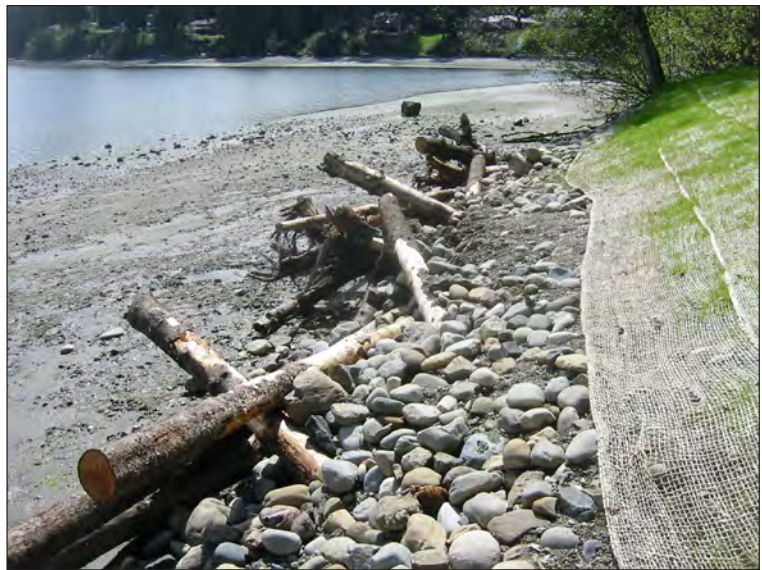
Figure 4. Frye Cove County Park, large wood and cobble slope stabilization, Eld Inlet, Washington.
