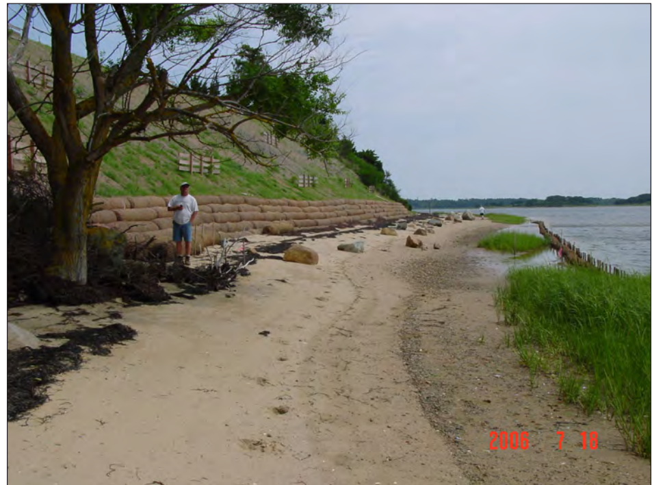
Figure 2B. The same coastal bank/bluff as shown in figure 2A showing a coir fiber roll revetment, that is, non-structural coastal armoring, that is preventing sand from eroding from the bank and feeding the fronting and adjacent beach and dunes.
