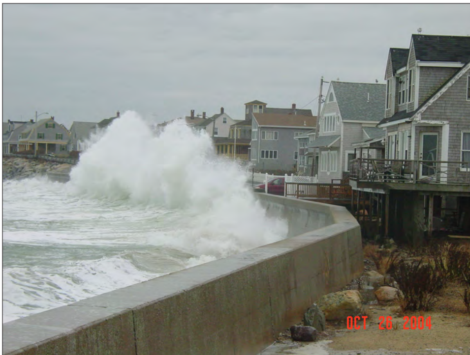
Figure 1. Vertical concrete seawall with toe stones protecting waterfront buildings from the direct impact of storm waves along the South Shore of Massachusetts.
