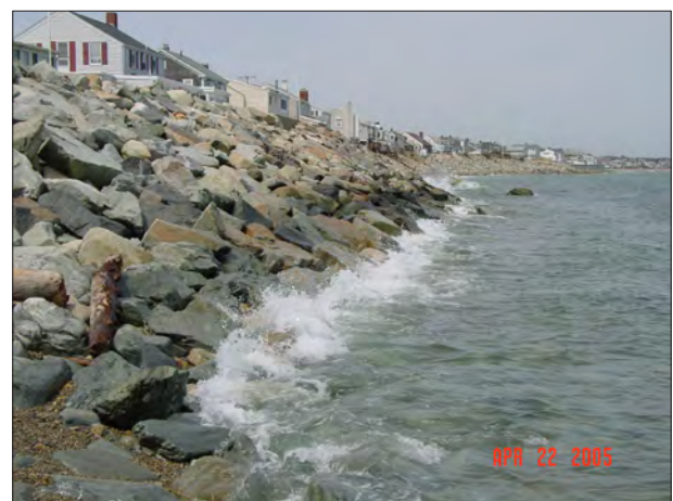
Figure 3B. The same coastal bank/bluff along the South Shore of Massachusetts (shown in fig. 3A) now structurally armored. As a result of 'passive erosion' and source sediment impoundment, the fronting beach has completely eroded away.
