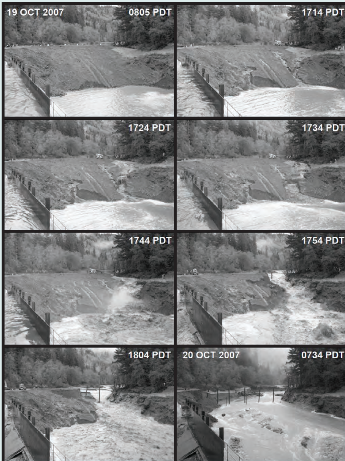
Figure S2.1. Breaching of the temporary earthen coffer dam on October 19–20, 2007, at the site of the manually removed Marmot Dam in northwest Oregon. Note the seepage and mass failures on the downstream face of the dam by 1714 Pacific daylight time (PDT). Incision downward into the coffer dam was nearly complete by 1804 PDT, and nearly all the coffer dam structure had been removed by 0734 PDT the next morning
