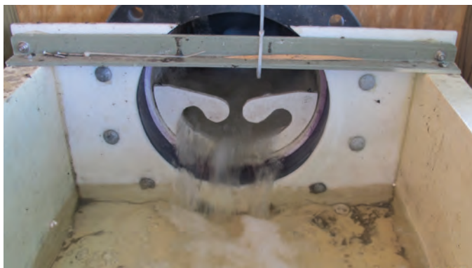
Figure 8. A static mixer assembly at U.S. Geological Survey bridge-deck-monitoring station on State Route 2A in Boston (422108071052501) in eastern Massachusetts, 2014–16. Location of station is shown on figure 1.
