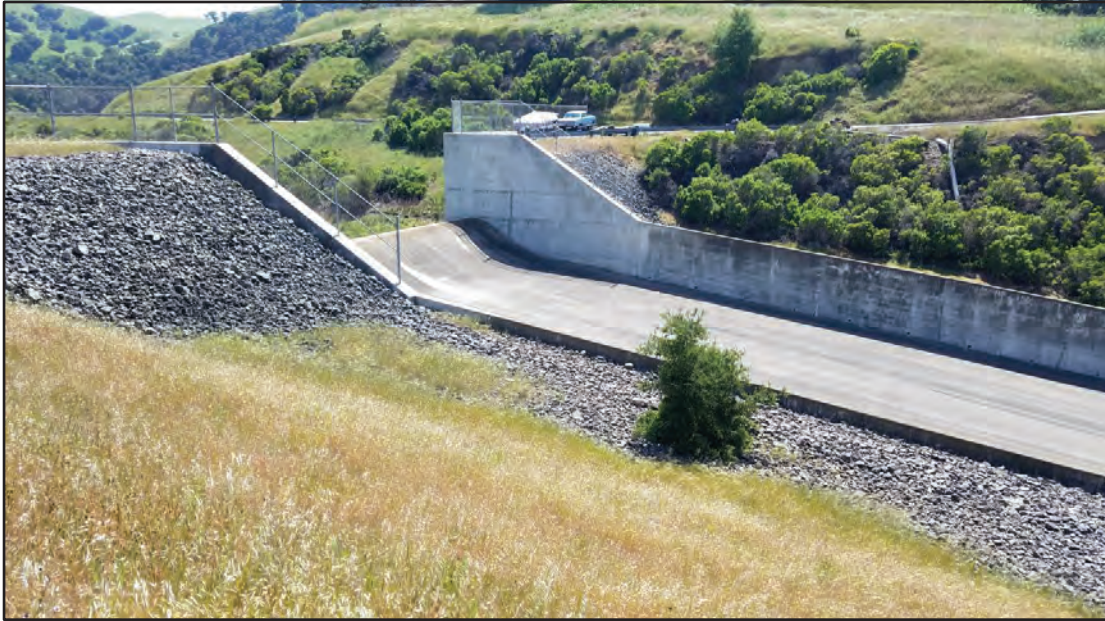
Figure 2. Spillway at the San Antonio Reservoir, California (photograph by Mathieu D. Marineau, U.S. Geological Survey, April 2018).
