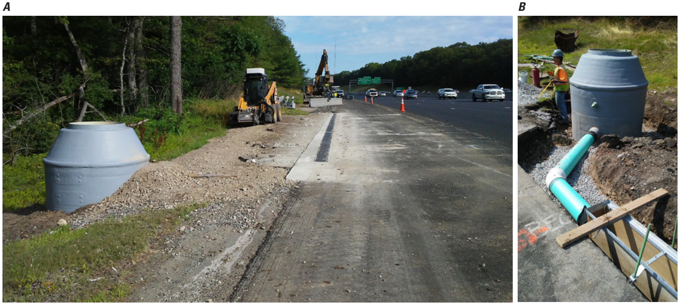
Figure 4. A, B , Photographs of the installation of the trench and metering manhole near the dense-graded hot-mix asphalt (HMA) at U.S. Geological Survey station 421650071120401, on Interstate 95 near Needham, Massachusetts, 2018. Station location shown on figure 1 . Photographs by Henry L. Barbaro, Massachusetts Department of Transportation, used with permission.
