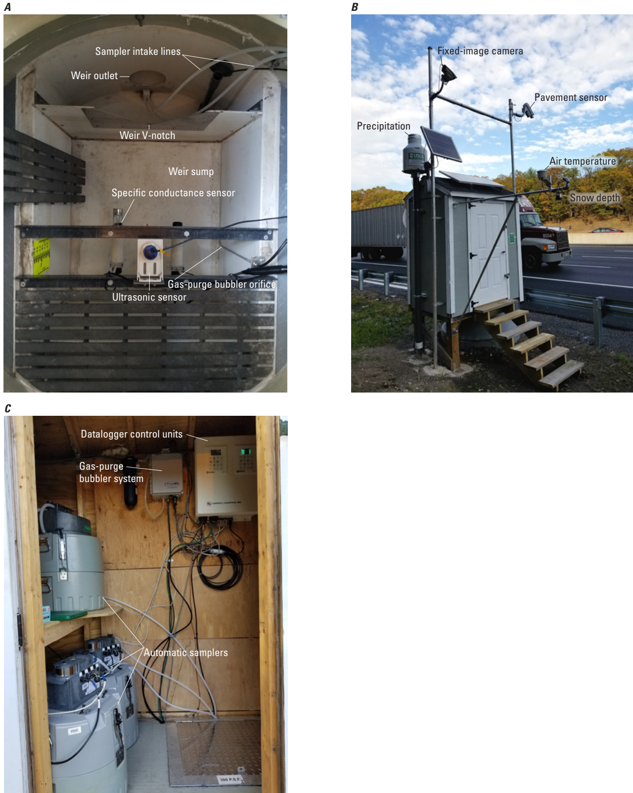
Figure 5. A, A top-down view of the weir box in the metering manhole, B, the highway monitoring station shelter adjacent to open-graded friction course (OGFC) pavement, and C, the instrumentation inside the monitoring shelter at U.S. Geological Survey station 421652071120601 on Interstate 95 near Needham, Massachusetts, 2018. Station location shown on figure 1 . Photographs by the U.S. Geological Survey.
