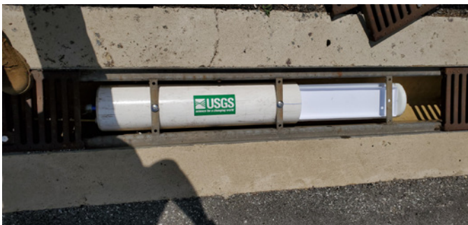
Figure 7. Photograph of the automatic dry-deposition sampler, with the collection tray in the open position, installed in the trench on Interstate 95 at USGS station 421652071120601, near Needham, Massachusetts, 2020.
