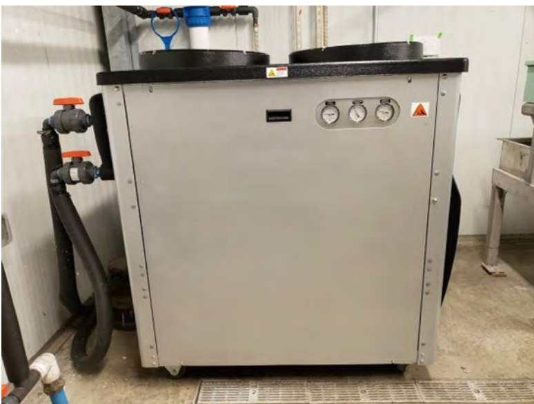
Figure 19. In-line water chiller.
