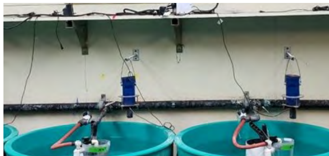
Figure 32. Automatic vibratory attached overhanging hatchery tanks.
