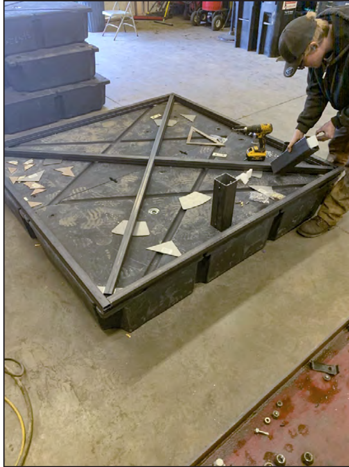
Figure 1. Construction of floating base and supports of bait delivery platform. Photograph by James Wamboldt, U.S. Geological Survey.
