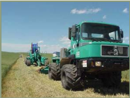
Photographs showing plowing and pulling to put minor pipelines in the ground in order to disturb much less ground and vegetation than excavating and trenching. Photographs by Bureau of Land Management.
