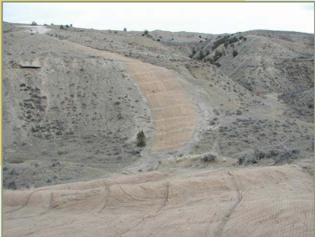
Photograph showing erosion blankets placed over a steep hillside as a cost-effective soil stabilization method. Photograph by Bureau of Land Management.
