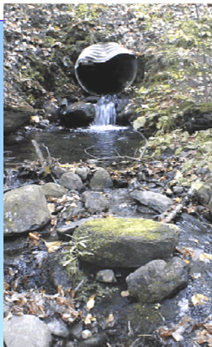
Above: culverts block fish migration and fragment thousands of kilometers of stream habitat
