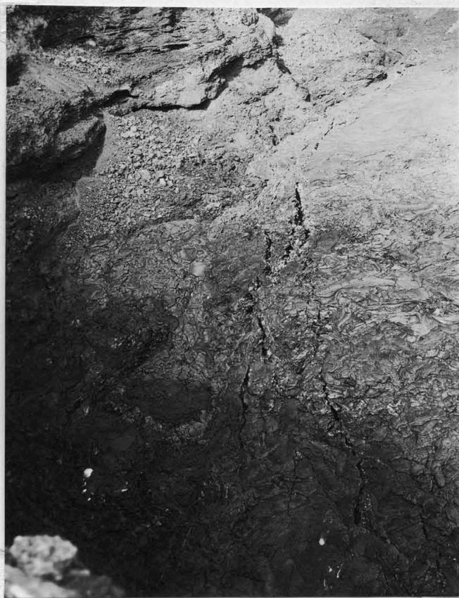
2. Cracks along S.W. wall, from S.S.W.
