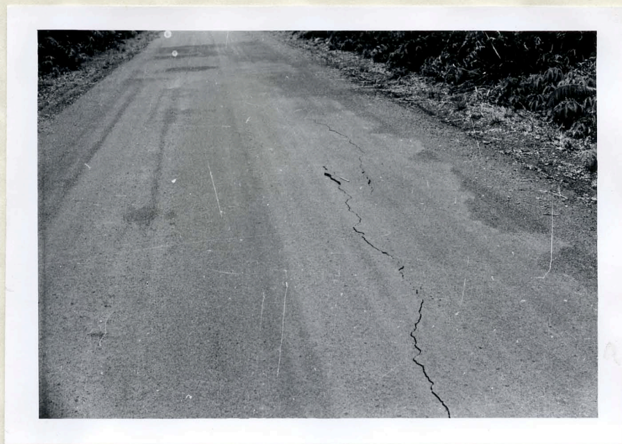
Cracking along Chain of Craters road.
