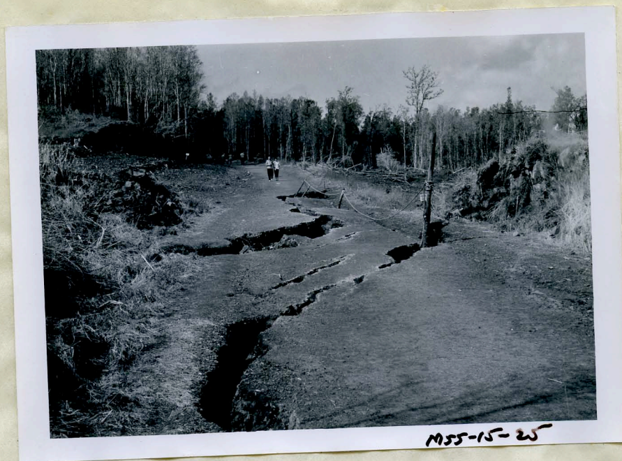
M55-15-25 Cracks in road at Nii's house, about June 15, 1955.
