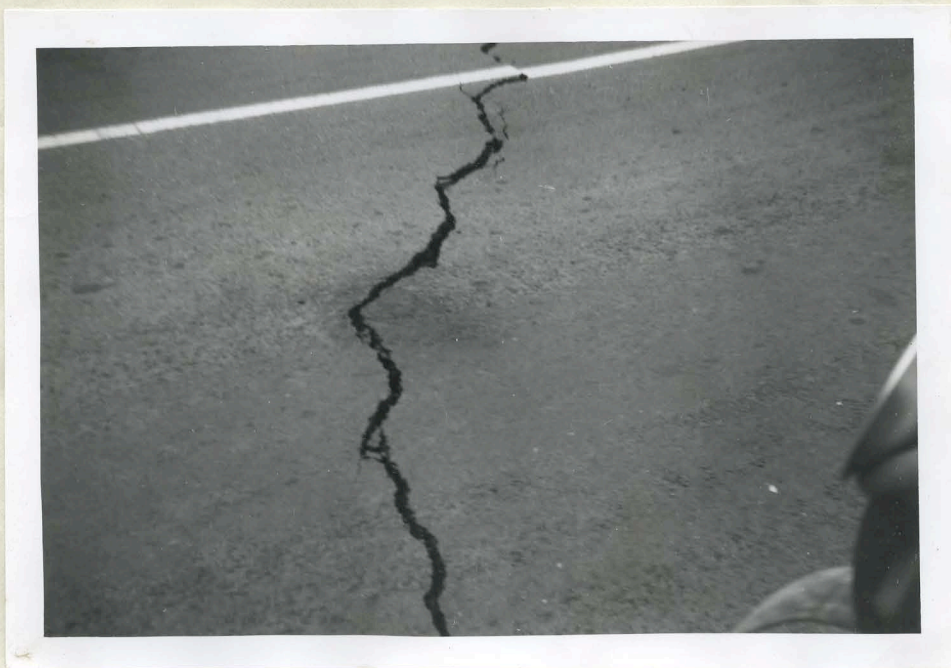
Crack in highway ca. 1/8 mile NE of Park headquarters, opened by earthquake at 16:02 on March 27, 1955.
