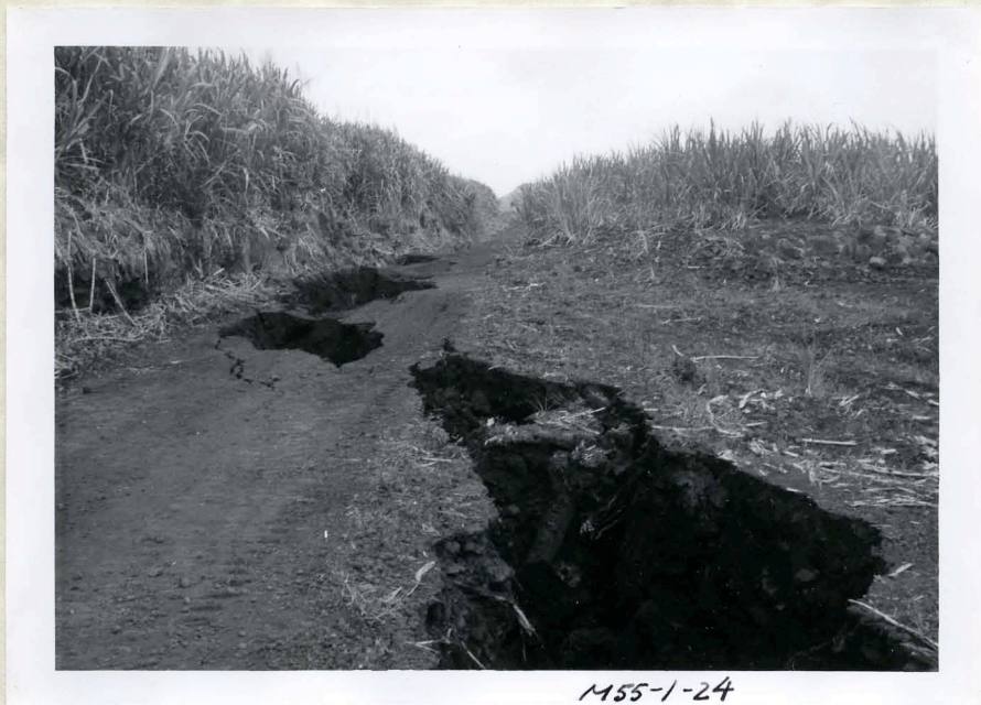
M1-24 Cracks along railroad bed road near base of Kaholua o Kahawali hill; 11:15, Mar. 2, 1955.
