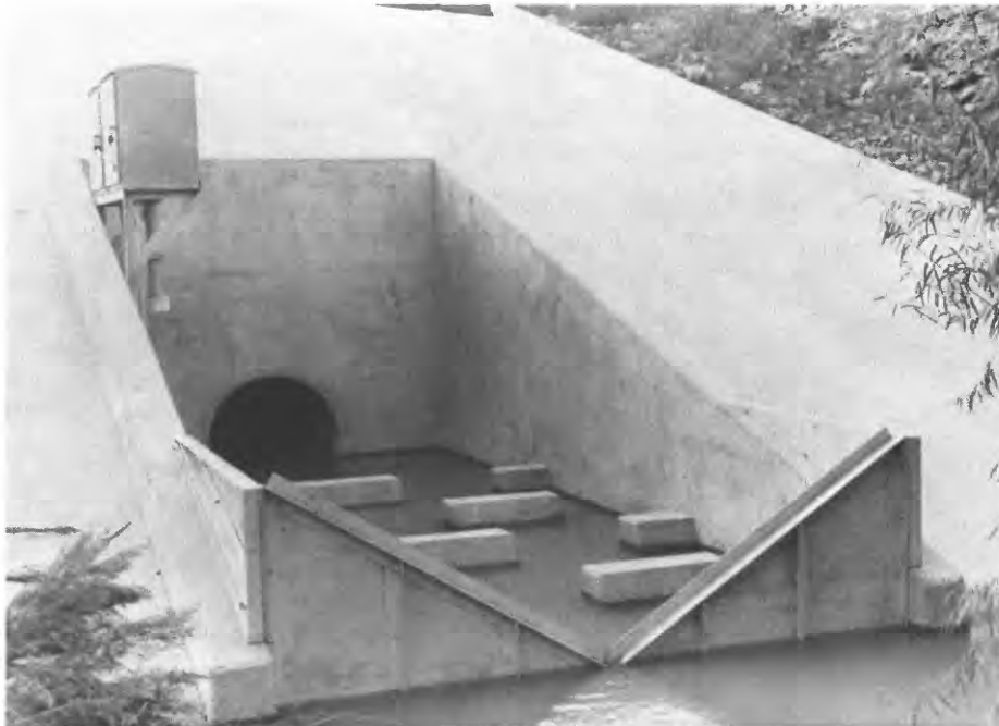
B. Outflow control structure for Pond 1 at Barton Creek Square Shopping Center
