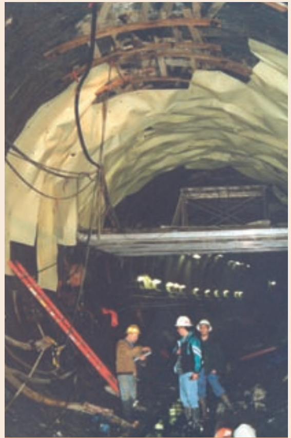
The 23-ft. diameter tunnel at the transmissive fracture zone. Note the roof instability and plastic sheeting used to divert ground-water seepage.
