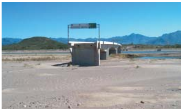
Post-Hurricane Mitch remnants of a newly constructed highway bridge across the Río Choluteca north of Choluteca. The bridge was designed to convey floodflows through the main span.
