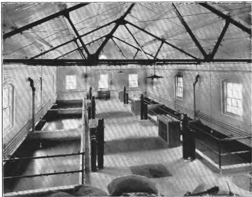
B. OPERATING FLOOR AND RAPID SAND FILTERS OF THE CHINCHILLA FILTRATION PLANT, SCRANTON, PA.
