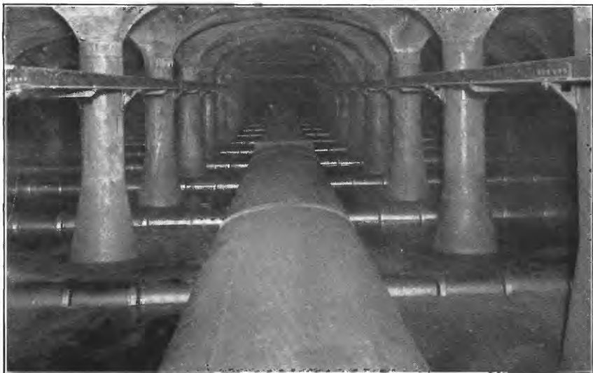
A. MAIN COLLECTOR AND LATERALS BEFORE SAND AND GRAVEL WERE PUT IN.
