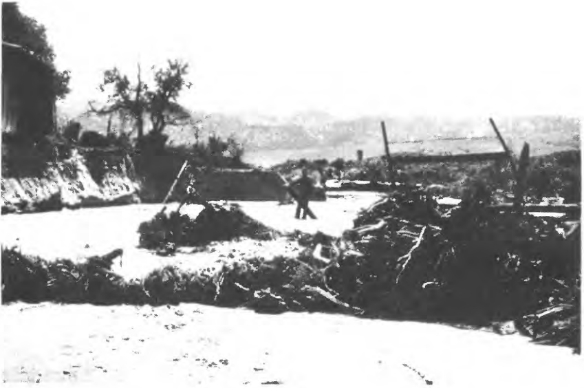
FIGURE 14.--Lateral migration of Cañada de los Alamos near Kinsey Ranch during February and March 1978. Channel receded 25 ft on left bank exposing pipeline to pumphouse. Original soil deposited on pipe indicates a maximum stream depth of about 3 ft near pipeline.
