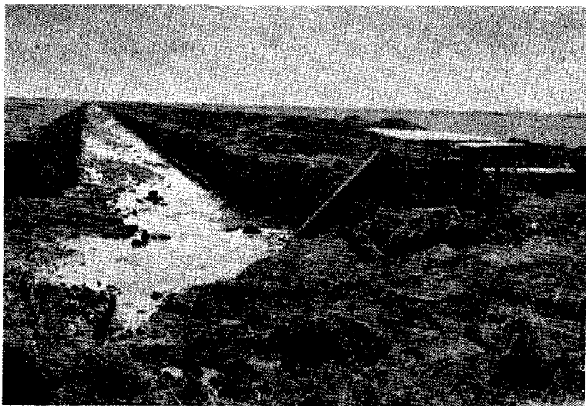
Figure 92. — Water control facilities in the upper Everglades. Main canal of East Shore Drainage District, under construction near Belle Glade; part of channel still to be excavated and spoil material to be graded to form a dike. Canal was excavated to the rock surface in 9 ft of muck soil; pump was a temporary installation for construction period; August 1944.
